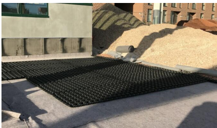
The drainage element Floradrain® FD 60 neo is laid onto the Protection Mat ISM 50.
